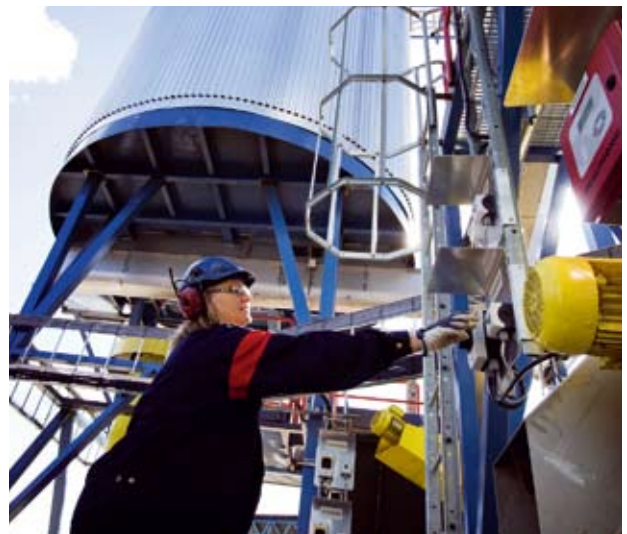
In Storuman, Skellefteå Kraft has developed a one-of-a-kind, next-generation bioenergy combine with an energy efficiency of 98 per cent.
